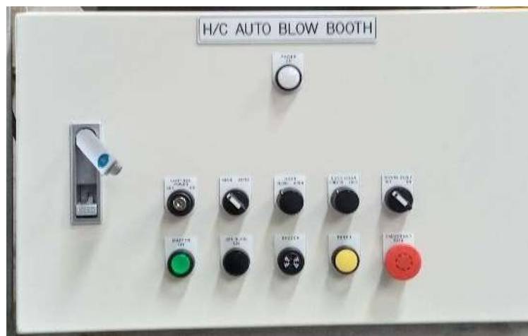
Gambar 1. 5 Panel Auto Blow Booth
