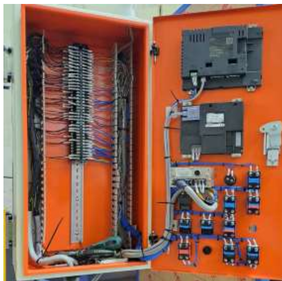
Gambar 2. 4 Wiring panel Auto Laser Marking MC
