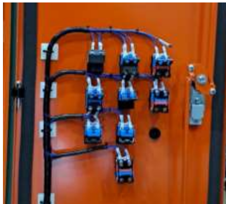
Gambar 2. 14 Wrapping spiral kabel panel Lifter Pallet Conveyor
