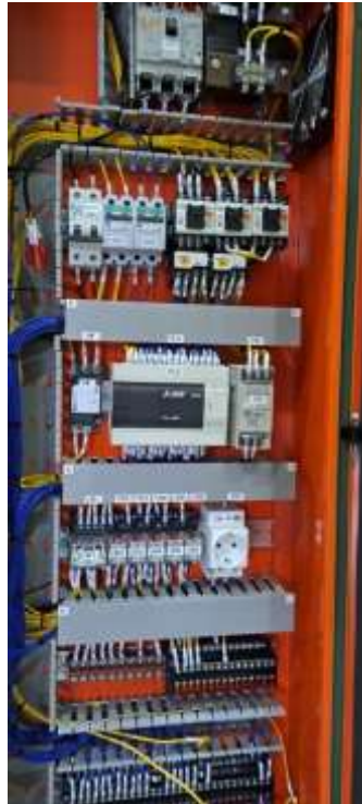
Gambar 2. 13 Wiring kabel panel Lifter Pallet Conveyor
