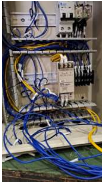
Gambar 2. 11 Wiring kabel panel Pokayoke Air Micro
