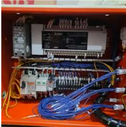
Gambar 2. 3 Wiring kabel panel Pokayoke Tigtening Device
