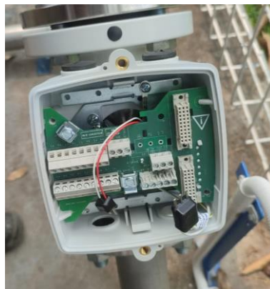
Gambar 2. 7 wiring Sensor Flowmeter PT. Coca Cola Botling Indonesia
