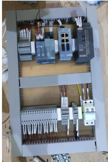
Gambar 2. 4 Wiring Panel Deepwell PT. Coca Cola Botling Indonesia
