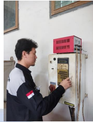
Mengatur Open Furnace 02
