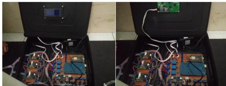
Gambar 4. 6 Hardware elektrik kontrol monitoring LPJU
