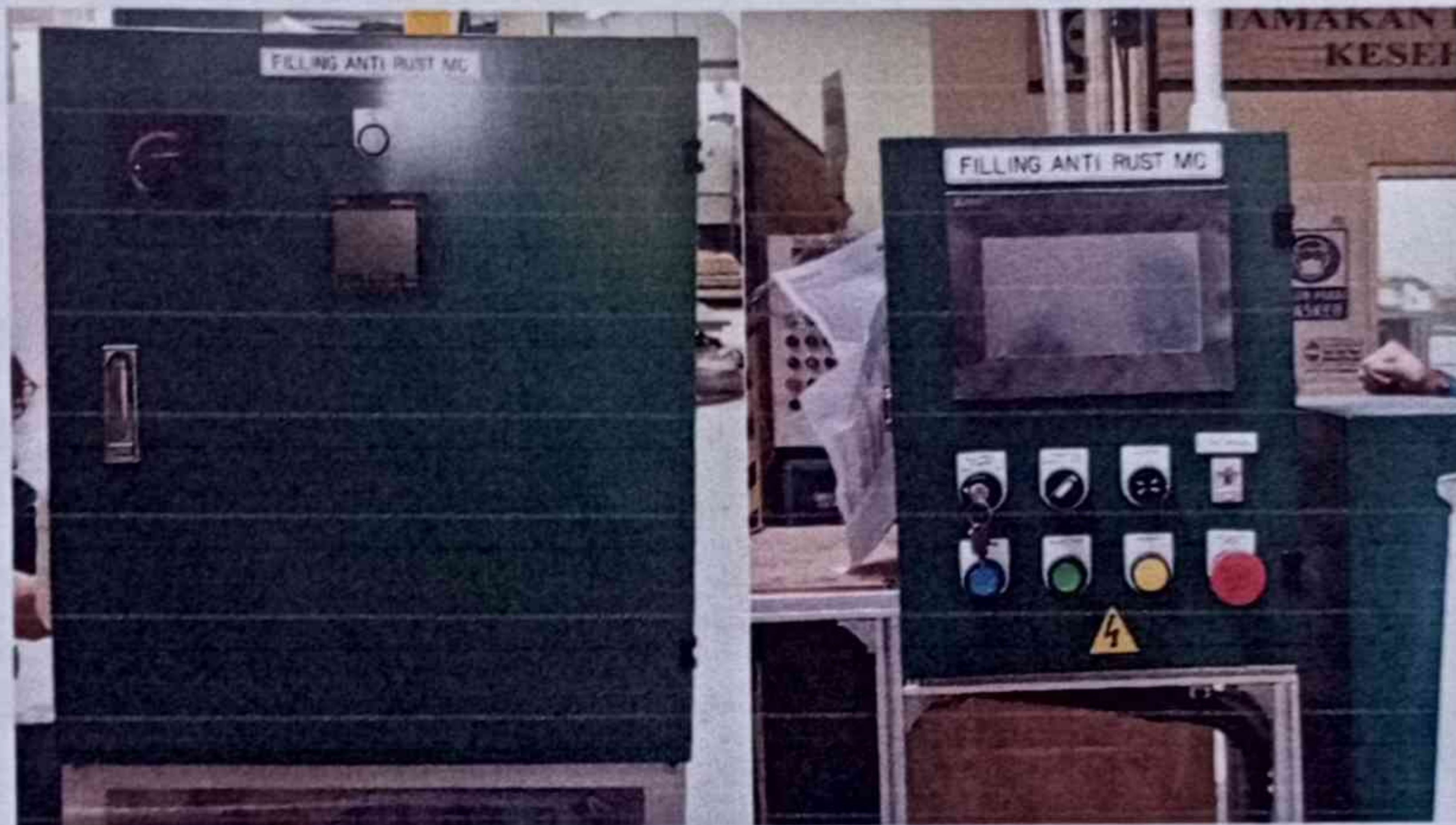
Gambar 1. 13 Panel Mesin Filling Antirust
