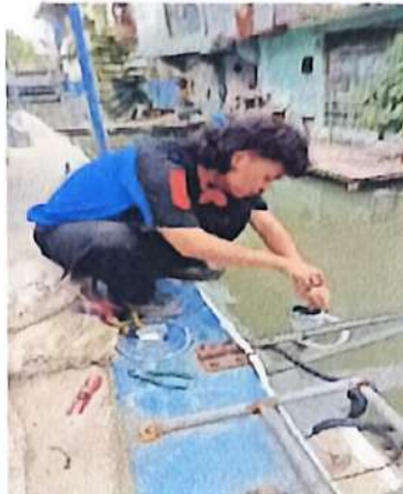
Gambar 2. 7 Instalasi Sensor Banjir
