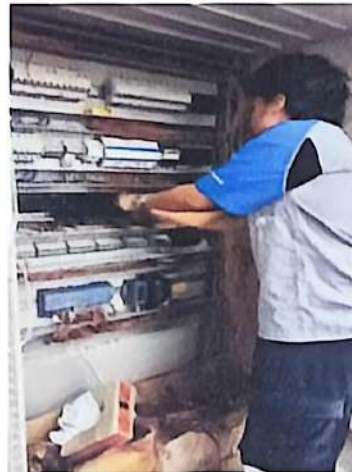
Gambar 2. 1 Wiring Panel PT. Sampora Manufacturing Indonesia
