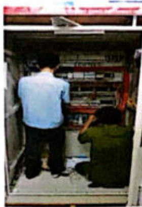
Gambar 2. 1 Wiring Power Panel Water Treatment Plant 4
