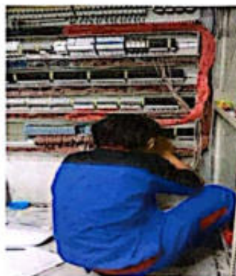
Gambar 2. 2 Wiring module PLC Siemens Simatic ET200-SP
