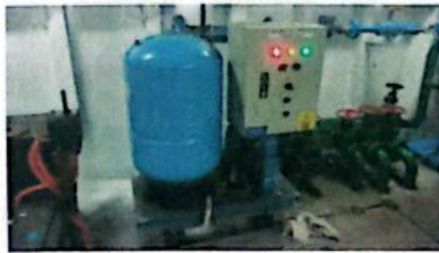
Gambar 2. 8 Commissioning Sea Water Pump
