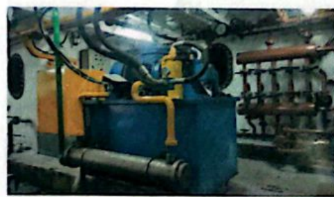
Gambar 2. 6 Commissioning Power pack
