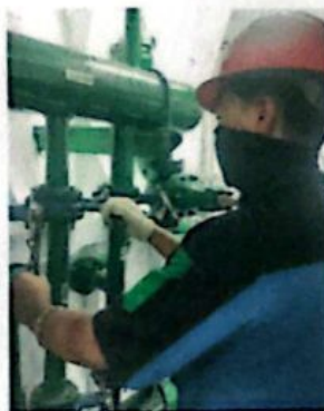
Gambar 2. 16 Proses Transfer Air Ballast
