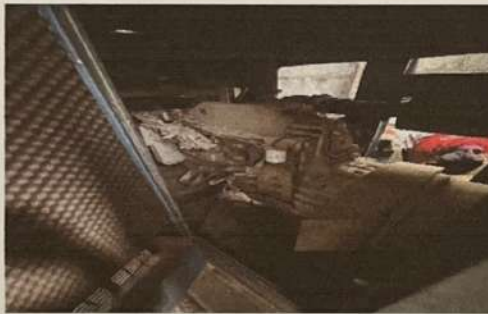
Gambar 2.6 Unit Mesin Genset (generator set)
