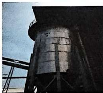
Gambar 2.16 Vertical Clarifier Tank (VCT)
