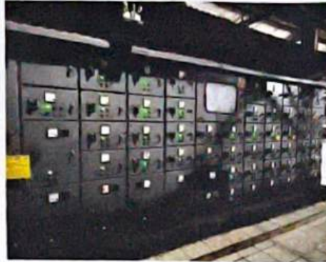
Gambar 2. 43 Panel Control machine karnel
