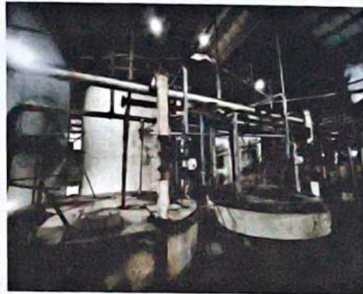
Gambar 2. 49 Continous Settling Tank (CST)
