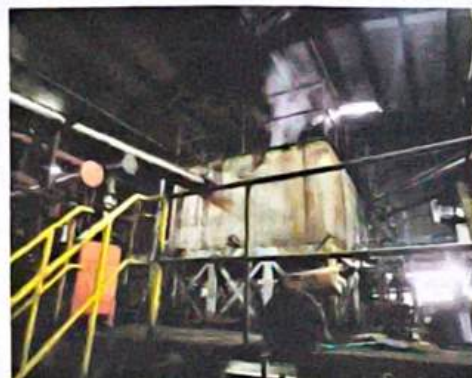
Gambar 2. 51 Balance & Hot Water Tank
