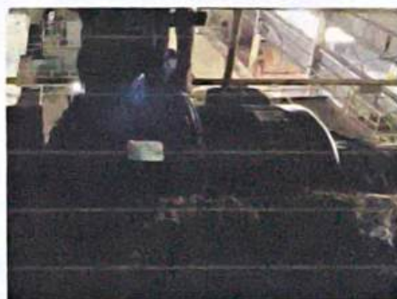
Gambar 2. 112 Motor 3 Phase di Threshing Station
