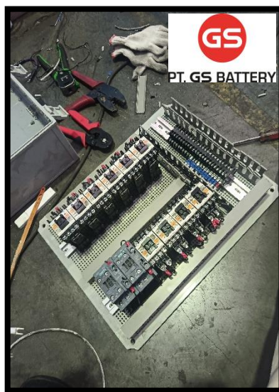
Gambar 7. Wiring Ulang Panel
