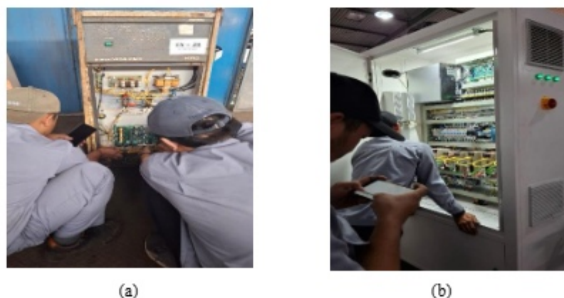
Gambar 2. 2 (a) (b) Perawatan Panel Box
