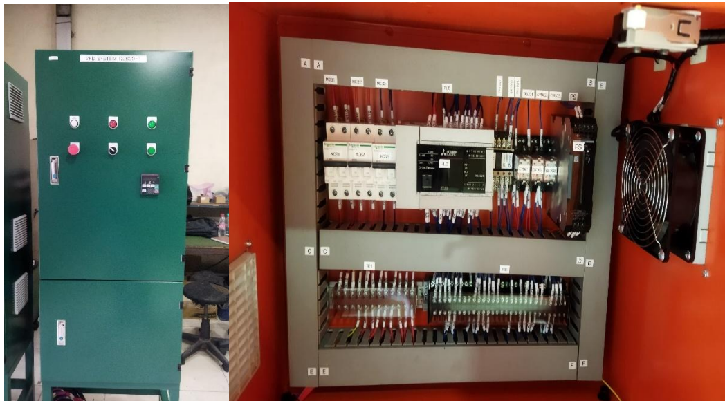
Gambar 1. 12 Panel VFD System
