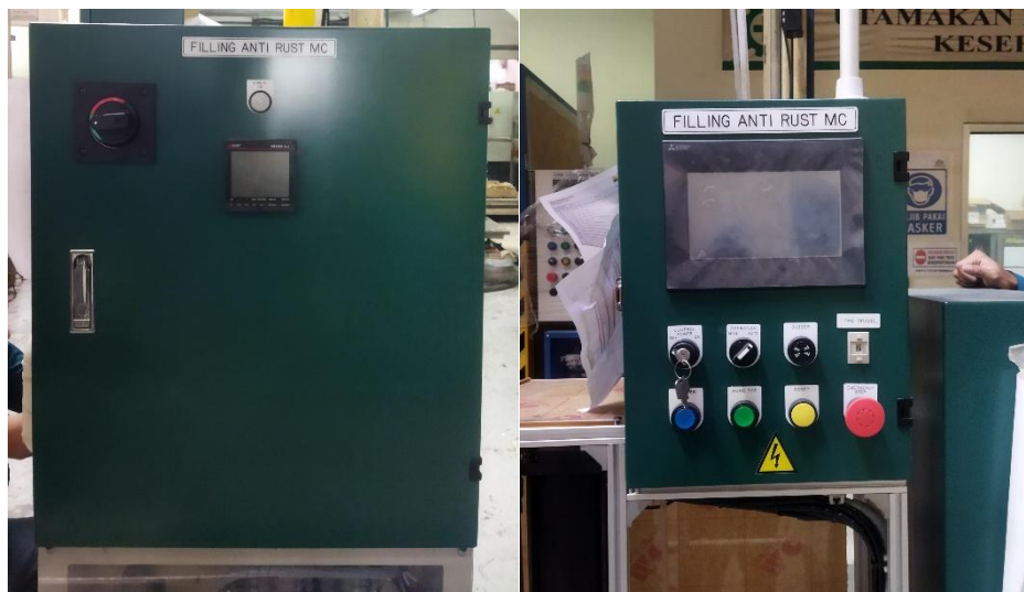
Gambar 1. 13 Panel Mesin Filling Antirust
