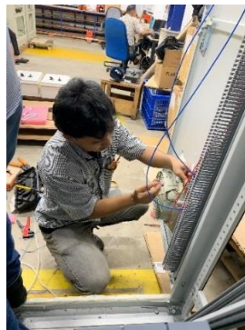
Gambar 2. 1 Terminal kabel blower fan PT. Darisa Intimitra
