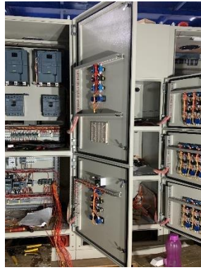
Gambar 2. 4 Wiring panel PT.ATMINDO
