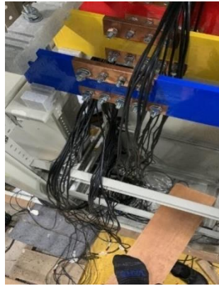
Gambar 2. 5 Terminasi power Incoming PT.ATMINDO
