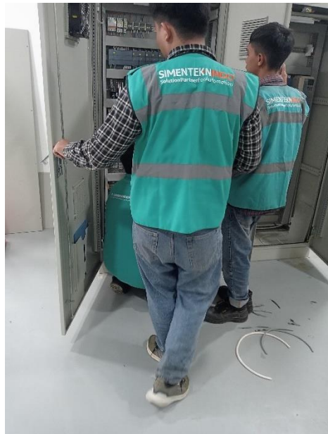
Gambar 2.15 Wiring panel PLC PT.FSD
