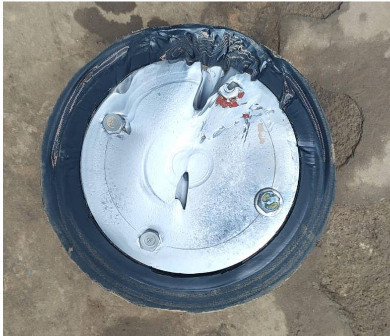
Gambar 2.6 Kerusakan Feed Valve
