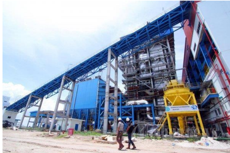
Gambar 1. 1 PT. PLN Nusantara Power Services Unit 3 PLTU Bangka
