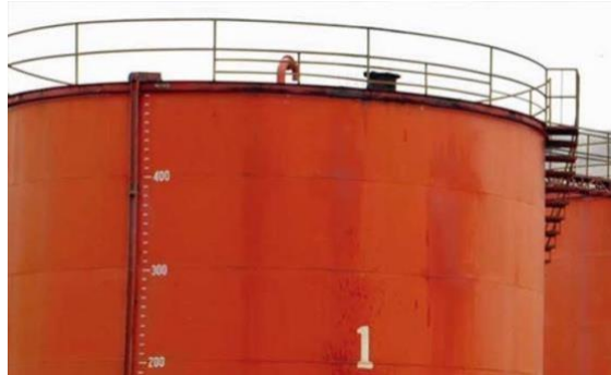
Gambar 20. Oil Storage Tank
