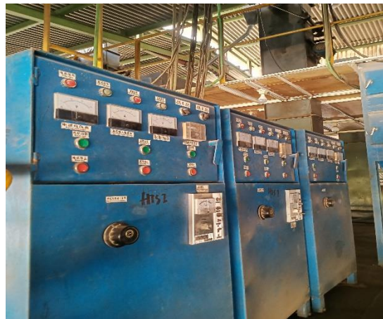
Gambar 2.6 Panel Kontrol Mesin HTS
