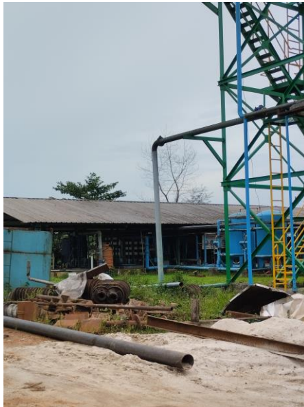
Gambar 2.11 Station Water Treatment Plant
