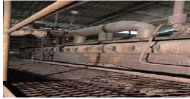
Gambar 2.40. Super Heater Boiler
