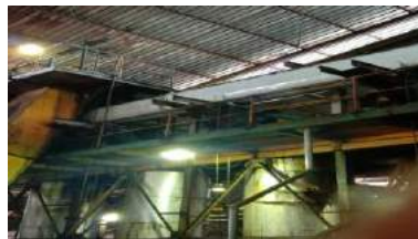
Gambar 2.20. Digester Feed Conveyor
