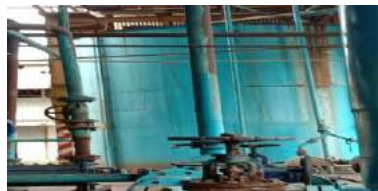
Gambar 2.38. Feed Water tank
