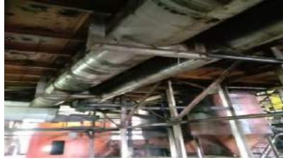
Gambar 2.24. Horizontal Cake Breaker Conveyor (HCBC)
