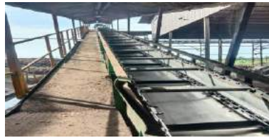
Gambar 2.16. Inclined Empty Bunch Conveyor (IEBC)
