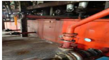
Gambar 2.27. Crude Oil Tank (COD)
