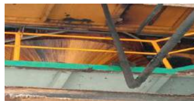
Gambar 2.28.1. Sludge Tank (Tangki Lumpur)
