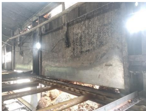
Gambar 2. 1 Pintu loading ramp
