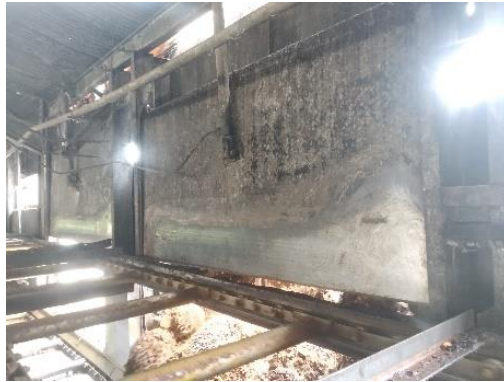
Gambar 2. 1 Pintu loading ramp
