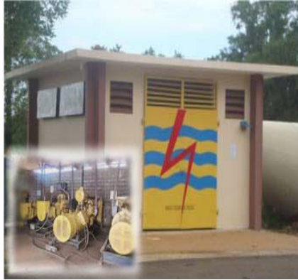
Gambar 1.3 ELECTRICITY ( PLN AND GINSET)
