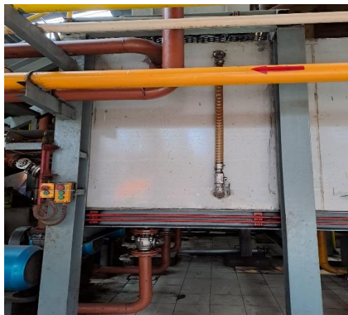
Gambar 1. 25 Dirty Oil Tank
