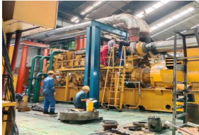
Gambar 2. 5 Corrective Maintenance Caterpillar Engine Generator
