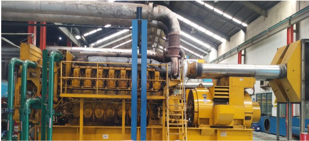
Gambar 2. 1 Caterpillar Engine Generator
