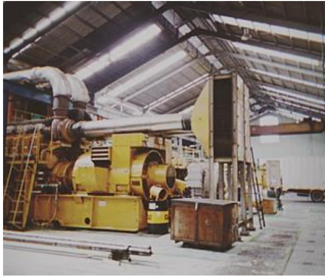
Gambar 2. 4 Predictive Maintenance Caterpillar Engine Generator
