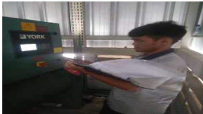
Gambar 2. 6 Dokumentasi Daily Ceklist Monitoring Harian Chiler York
