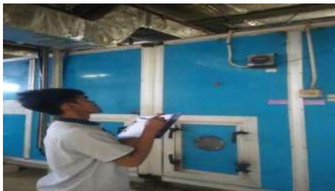
Gambar 2. 11 Dokumentasi Daily Ceklist Monitoring Harian AHU
