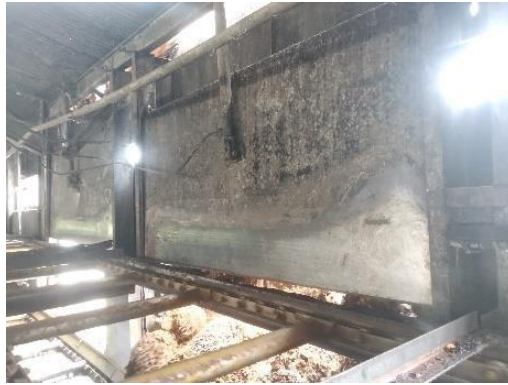
Gambar 2. 1 Pintu loading ramp
