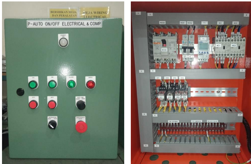
Gambar 1.16 Panel ON/OFF Electrical & COMP
