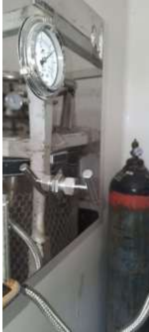
Gambar 2.8 Pengecekan saluran gas
