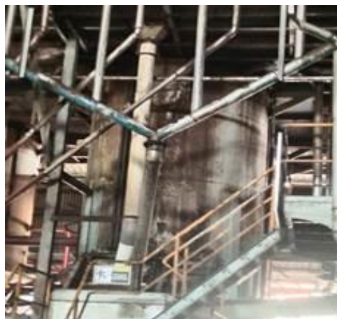
Gambar 2.8 Sand Trap Tank
