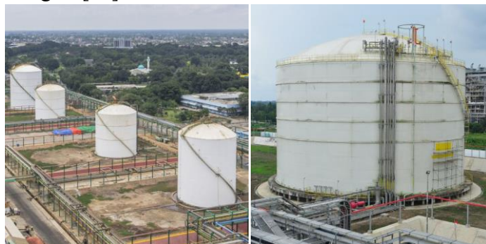
Gambar 1.19. Tangki Ammonia PT. Pusri Palembang [12]
