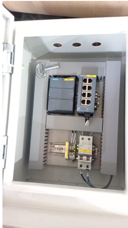
Gambar 2. 24 Hasil Wiring Panel Junction Box Repeater PT. Firmenich Aromatics Indonesia
