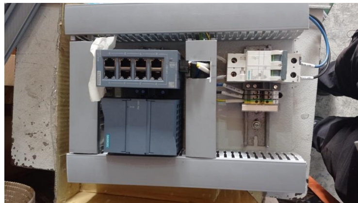
Gambar 2. 23 Proses Pengerjaan Wiring Diagram Panel Junction Box Repeater PT. Firmenich Aromatics Indonesia
