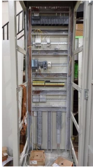
Gambar 2. 15 PLC Panel PT. Berkat Nirwana Teknik
