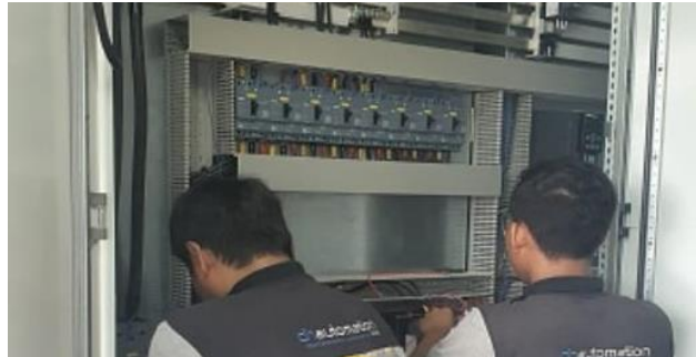
Gambar 1. 24 Control Panel Assy
