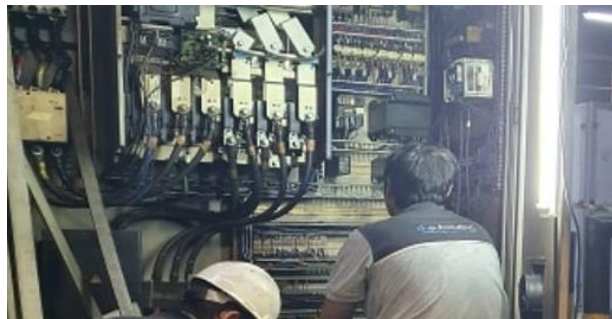
Gambar 1. 27 Control Panel Upgrade
