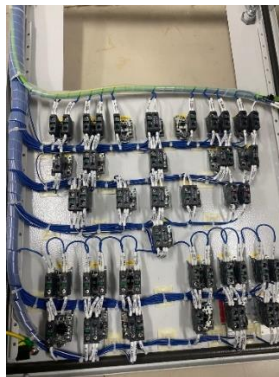
Gambar 2. 17 Perapihan Wiring I/O Panel OPR Curring
