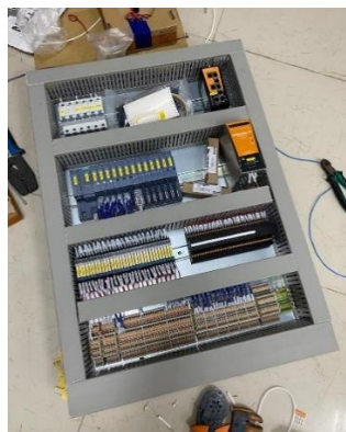
Gambar 2. 20 Wiring Panel Autoclave
