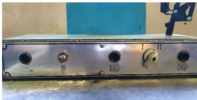
Gambar 4.2 Lampu Indicator rusak
