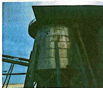
Gambar 2.16 Vertical Clarifier Tank
