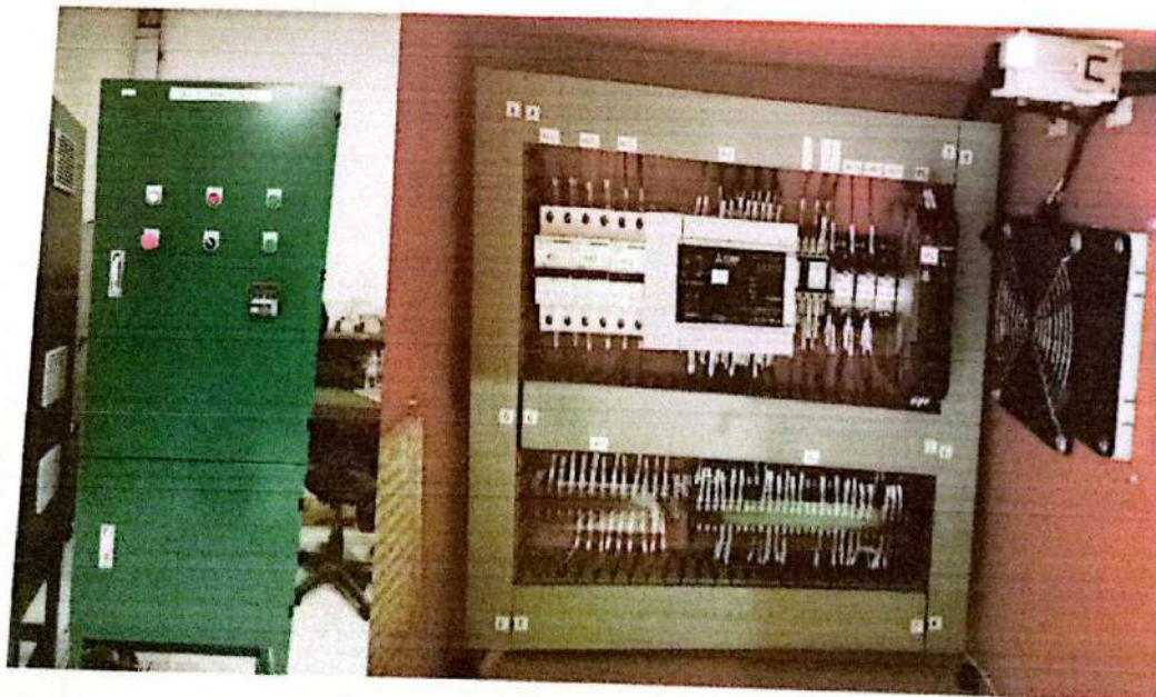
Gambar 1. 12 Panel VFD System
