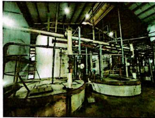
Gambar 2. 49 Continous Settling Tank (CST)
