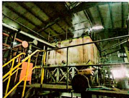
Gambar 2. 51 Balance & Hot Water Tank
