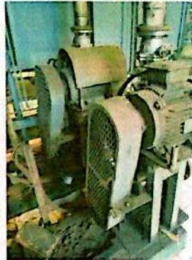
Gambar 2. 43 Motor pompa bak fit
