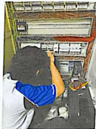
Gambar 2. 1 Wiring Panel Genset WTP PT.Nusa Cipta Indonesia
