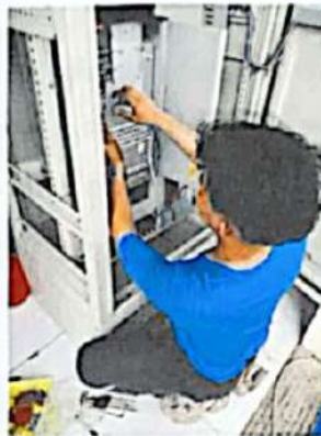
Gambar 2. 4 Site Upgrade Panel dan Terminasi
