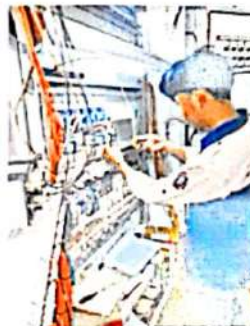
Gambar 2. 9 wiring panel MCC dan BOILER CELL 6
