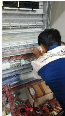
Gambar 2.1 Wiring Panel WTP PT. Nusa Cipta Indonesia
