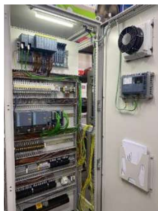
Gambar 2.11 Power UP Panel New MCWP IO Cabinet
