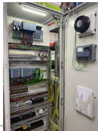
Gambar 2.10 Power UP Panel New Position ABB Building
