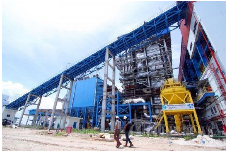
Gambar 1. 1 PT.PLN Nusantara Power Services Unit 3 PLTU Bangka
