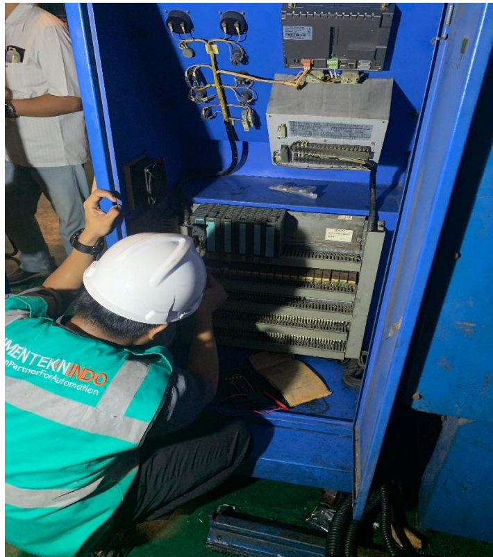
Gambar 2. 3 Penggantian unit CPU PLC di PT. Plasindo Bhama Prasasta
