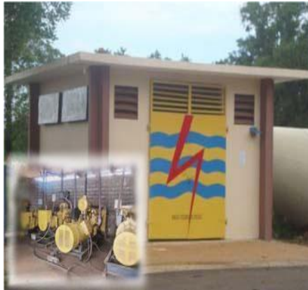
Gambar 1.11 ELECTRICITY ( PLN AND GINSET)
