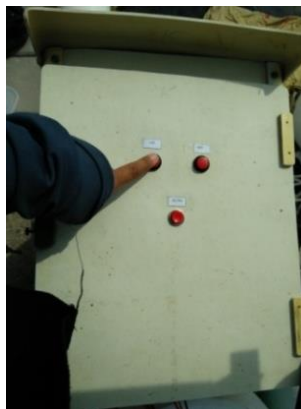
Gambar 4.30 Hasil pengujian push-button ON di box panel
