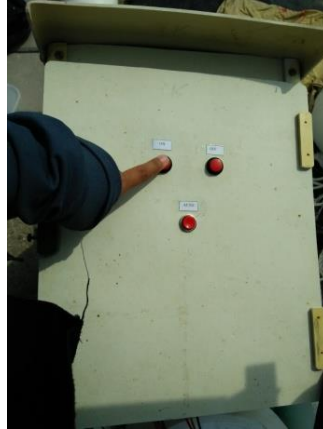
Gambar 4.36 Penyalan pompa mode manual ( push-button )
