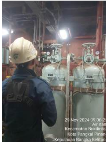
Gambar 2. 16 Pengecekan compressor system
