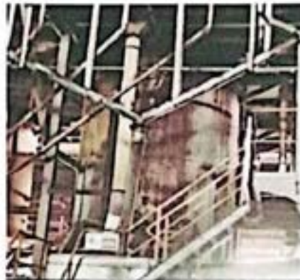
Gambar 2. 8 Sand Trap Tank
