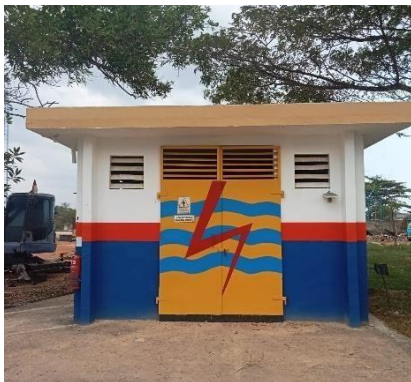
Gambar 1.4 Electricity ( PLN And Genset)
