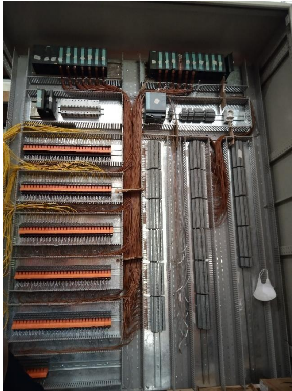
Gambar 1. 22 Panel TLPT PT. Andalan Furnindo
