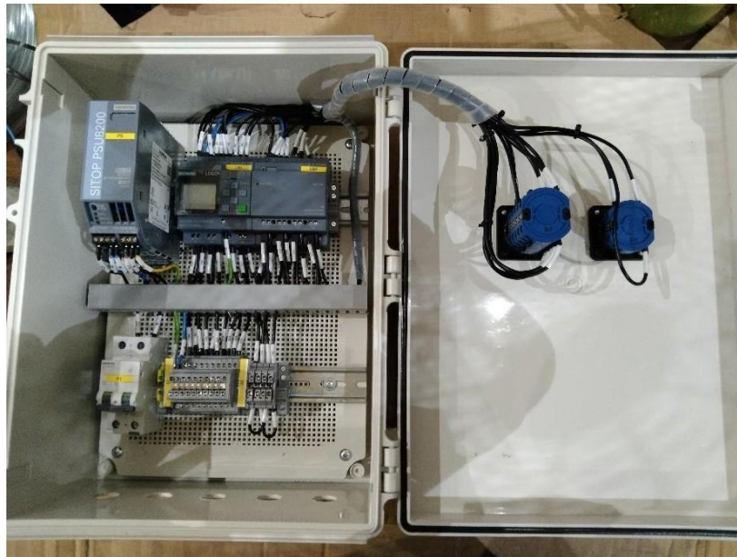
Gambar 1. 21 Panel control PT. Martin Supra Engineering
