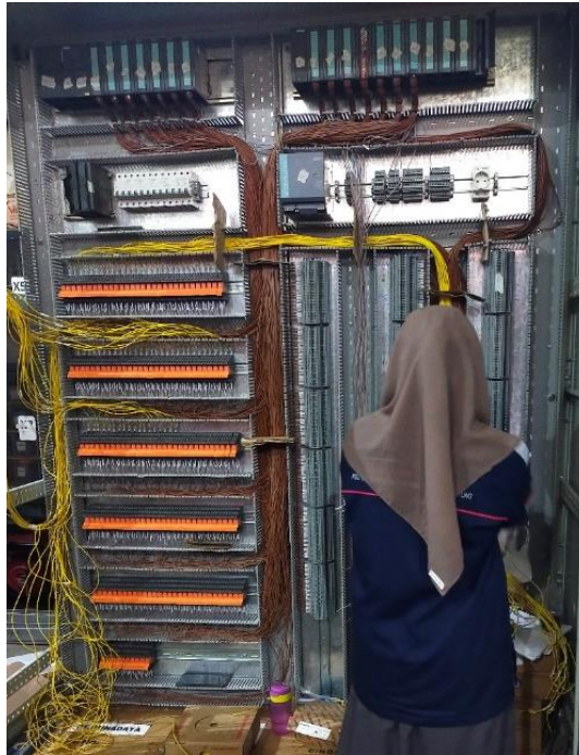
Gambar 2. 3 wiring panel TPLT project
