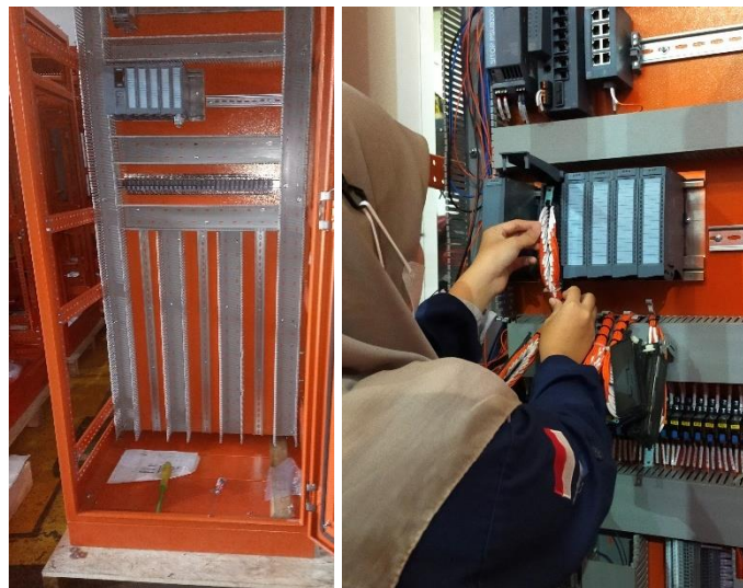
Gambar 2. 8 wiring panel PT. Borneo Indobara
